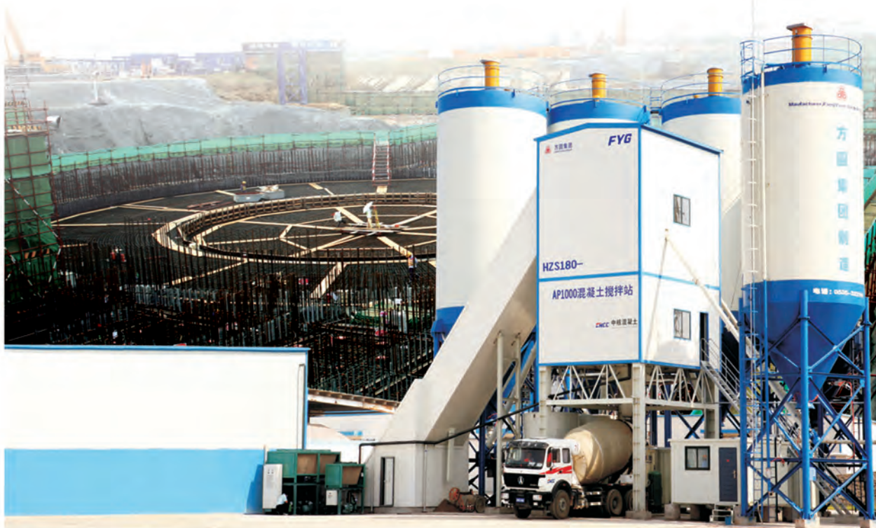
▲ Precooling concrete mixing plant
